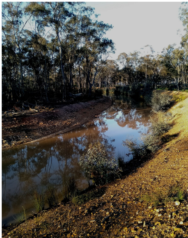
Flood mitigation works in the bush behind Dunolly hospital. Photo by Em Goldy
