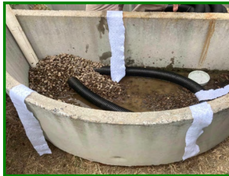
Wicking strips of geotextile placed before adding basalt as the bottom layer with a slotted drain pipe.
