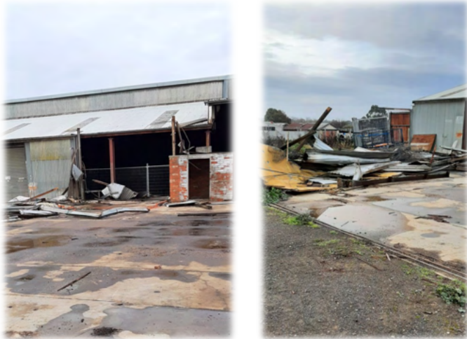
Photos taken last week showing the damage
